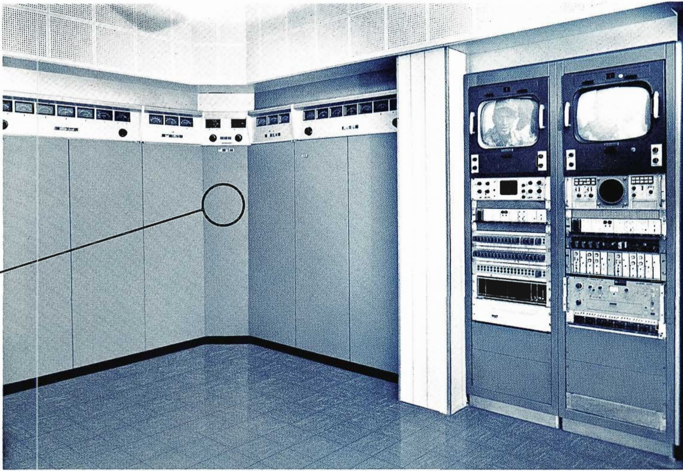
(Above) Visual input and monitoring racks are located next to one of the 25 kW amplifier cabinets.
