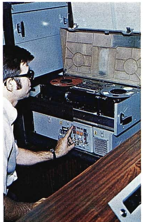
TPR-10 quad VTR's are drawer-mounted in van in front of video switching position.
