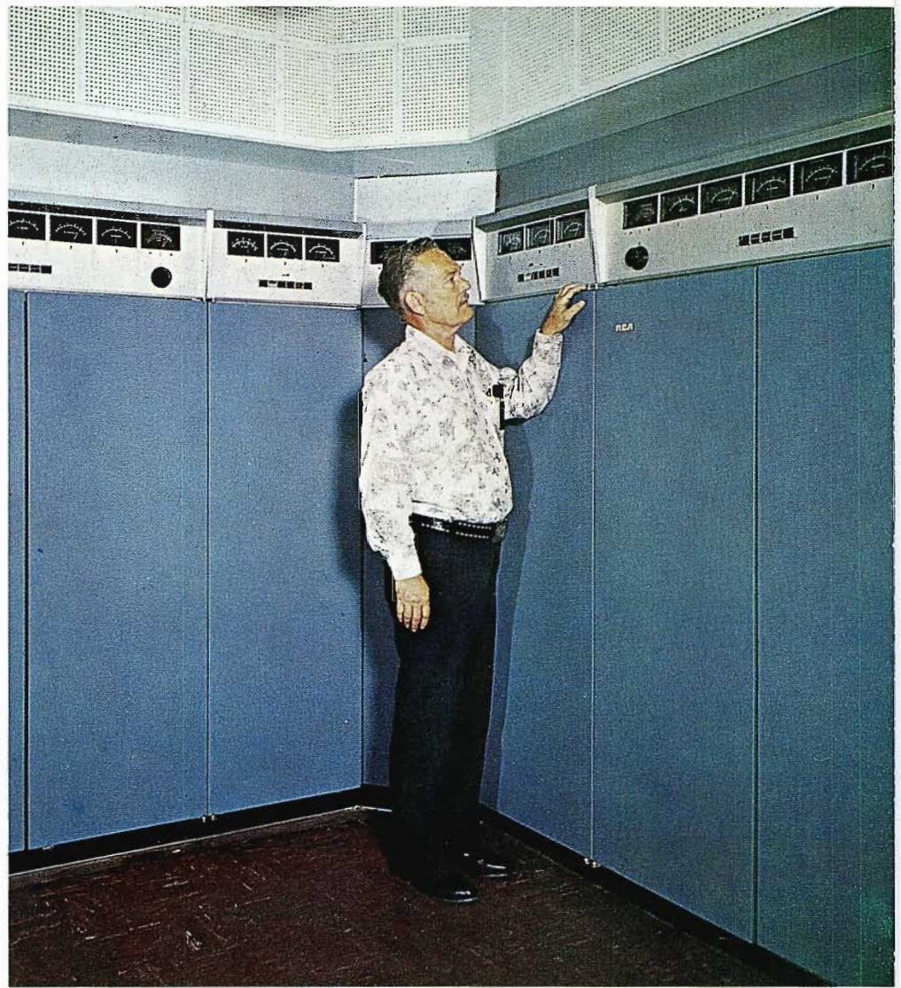
Transmitter Supervisor Bill Blacksher checks KTTV's 50 kW TT-50FH Transmitter.
